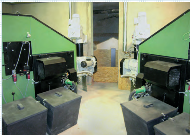
"St. Michael's Church" in Leipzig heats using two HDG Compact 100 units
