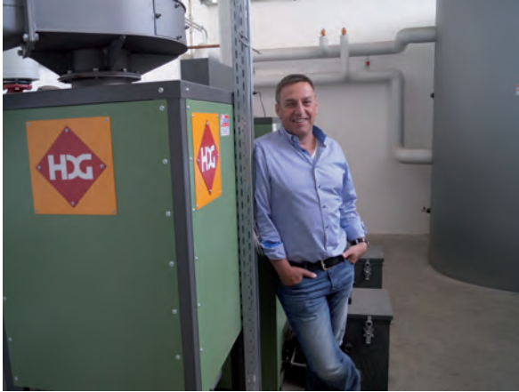
The First Competence Center of the company Unterreiner in the Lower Bavarian book is heated by a HDG Compact 150.
